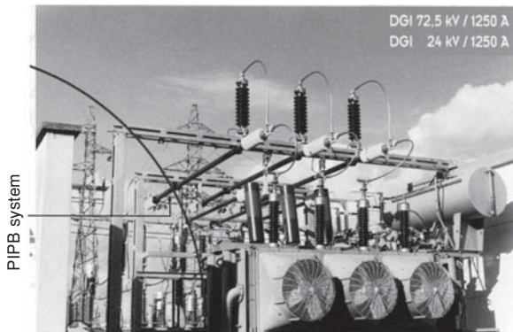
Figure 28.4(h) Layout of a 72.5 kV/1250A PIPB at a switchyard (Courtesy: MGC Technologie AG)
