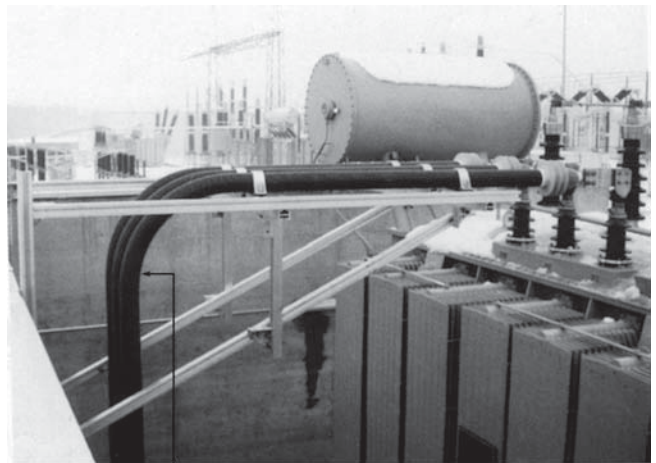
(g2) Connecting on the 24 kV/2500A transformer side
